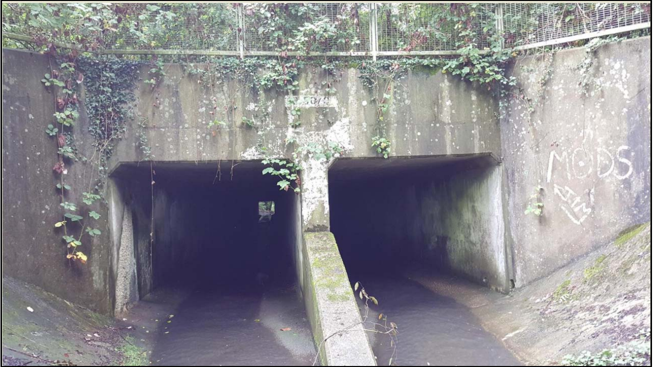
Figure 12: Twin box culvert beneath Wigley Bush Lane (Source: BB Surveys Ltd, August 2015)
