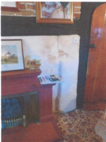
Fireplace in rear living room to be opened up – note damp chimney breast
