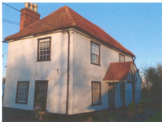
Sash windows to be repaired
