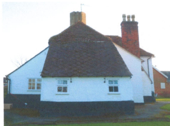
Lean-to roof and missing gutter
