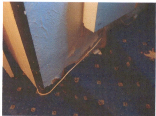
Damp plaster on second chimney breast
