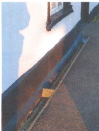
Gully formed in attempt to keep damp from brick plinth
