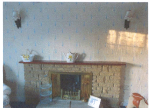
Fireplace in front living room to be replaced – note damp chimney breast
