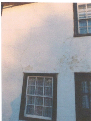
Surface deterioration of lime render
